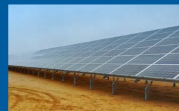
Mikhailovskaya solar power plant with
